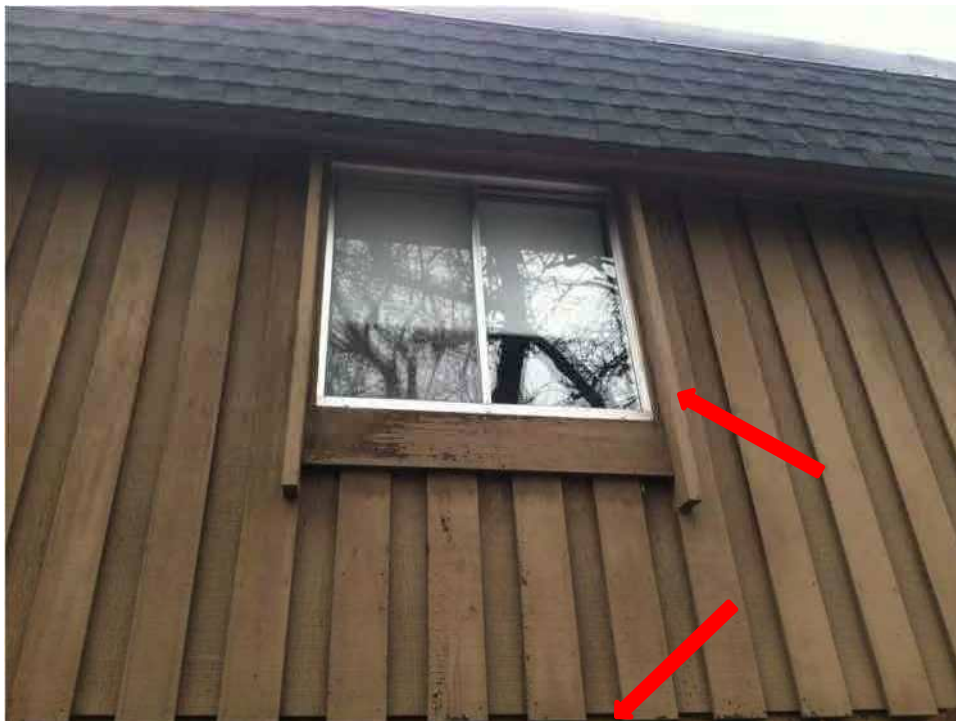
Photo 6 – Lead-Based Paint on Exterior Window Casing Boards & Lower Soffits
