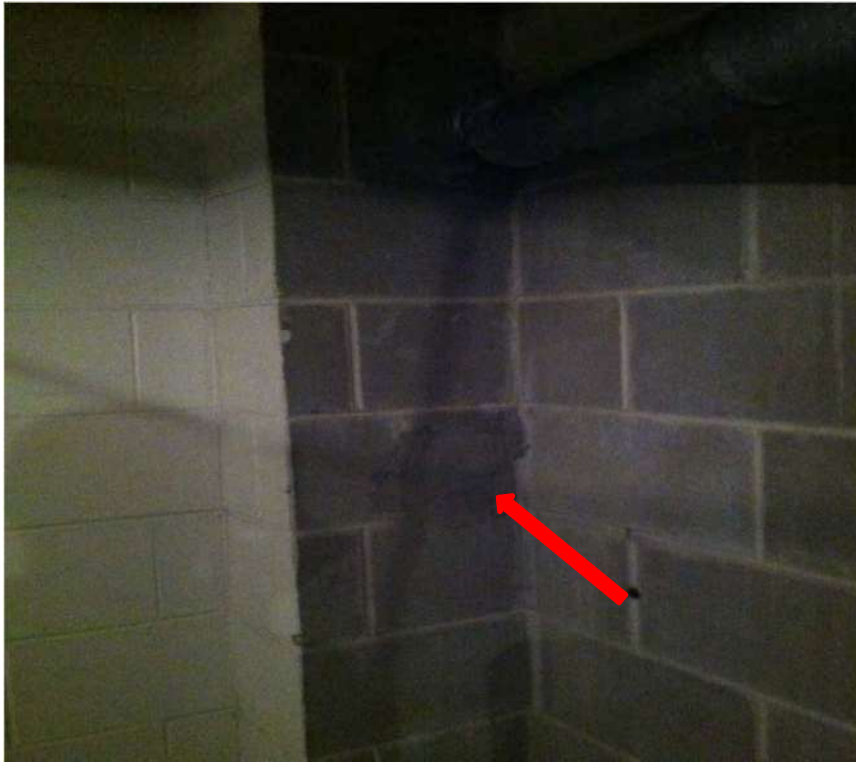
Photo 1 – ACM Packing on Old Chimney Flue Opening
