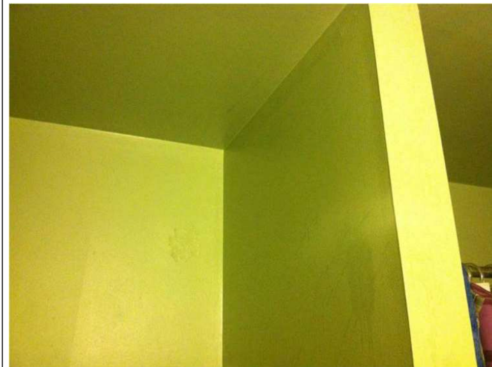
Photo 4 – ACM Joint Compound on Non-ACM Drywall
