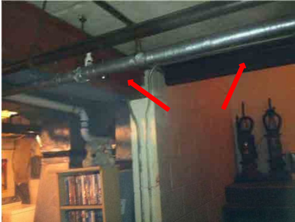
Photo 5 – Lead-Based Paint on Metal I-Beam & Angle Iron in Basements
